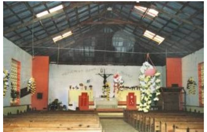
St. Bertin was both simple on the outside and inside, but adequate for the parishioners needs.
